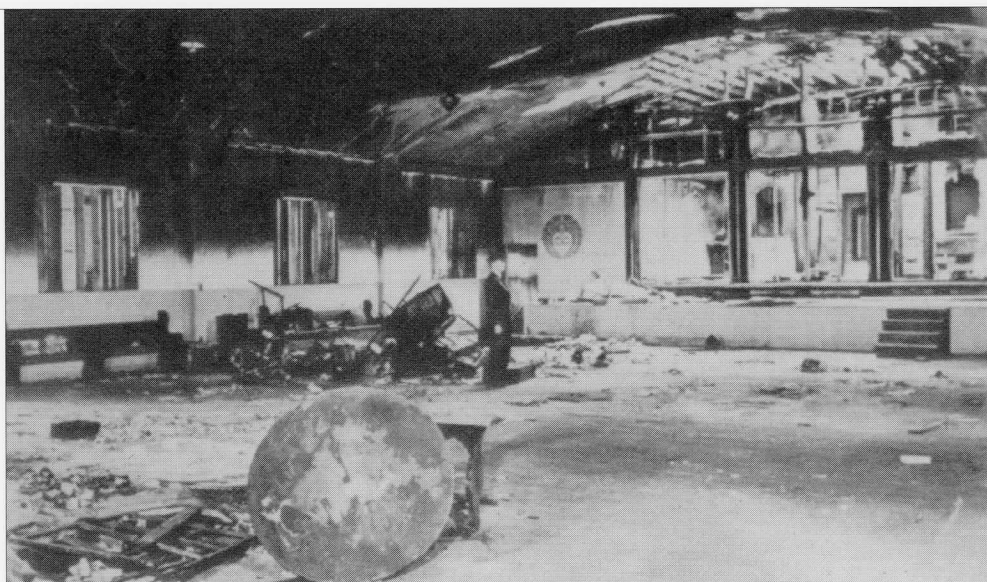
Hondo (sanctuary) of the San Diego Buddhist Church after it was damaged by fire in January 1943. Interned church leaders managed to lease the building to the USO, who paid a very low rent in exchange for repairing the building. The church was not returned until July 1947. Courtesy of BCA.
